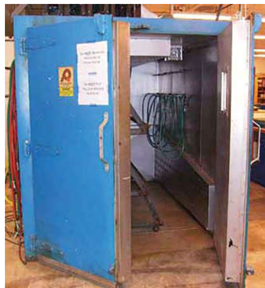
Figure 3-32. Walk-in curing oven.
